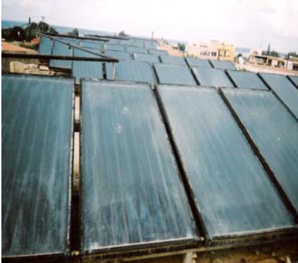
Figure 1. Solar collector field in the hotel Rethymno Village for solar cooling application
