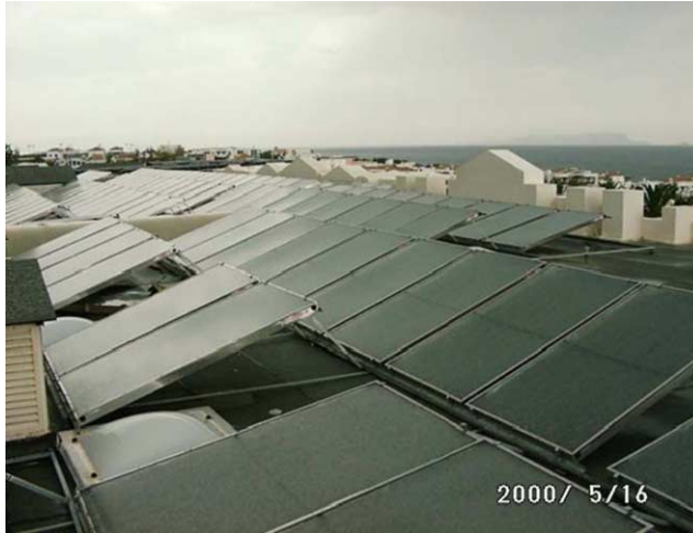
Fig. 7. Flat plate collectors' central solar system.
