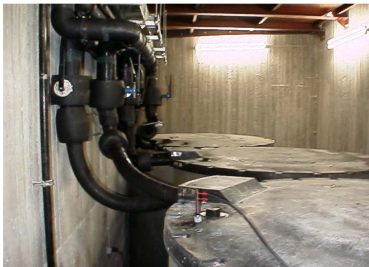
Picture 2 - AVAX building ice banks, Basement level (-3)
