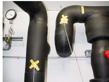
Picture 5 - PT100 temperature sensors, basement level (-3)
