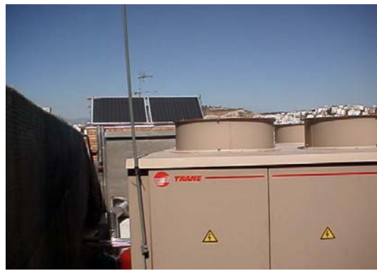
Picture 3 - AVAX building heat pump, roof
